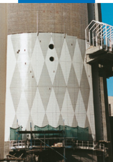
An example of an installation of klinker on concrete with Kerabond + Isolastic - New Telecommunication Tower - Kuwait City (Kuwait)
