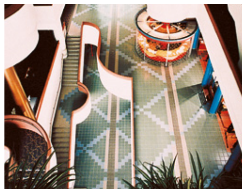
"Porcelain" quarry tiles laid with Kerabond + Isolastic - Civic Center - North York Ontario (Canada)
